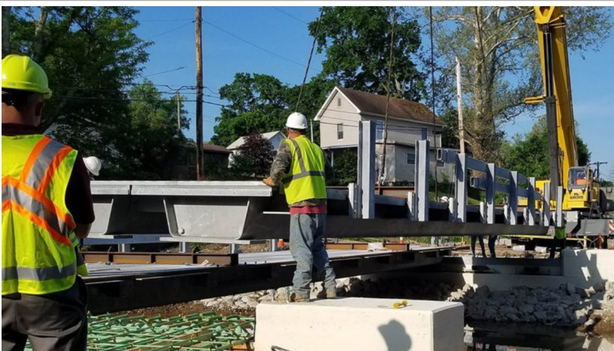
The press-brake tub girder modules for the Cannelville Road Bridge (Muskingum County, Ohio) were erected and positioned on their abutments in just 22 minutes.
