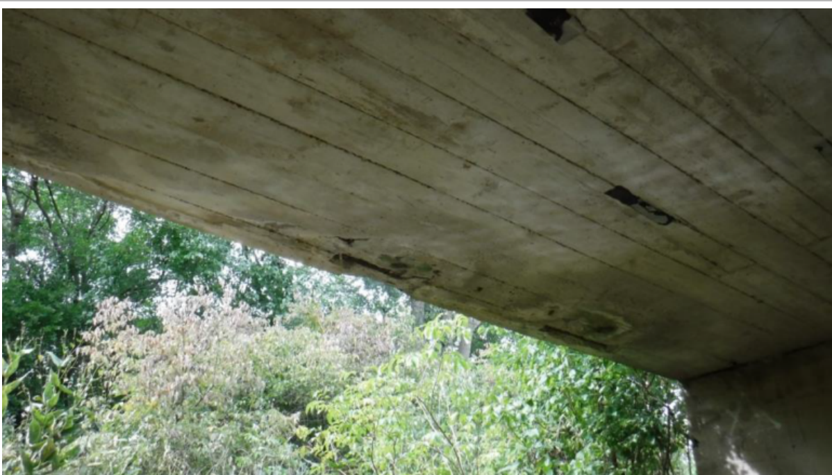
The Evans Mill Road Bridge is a reinforced concrete slab structure with a 35.4 sufficiency rating out of a possible 100.
